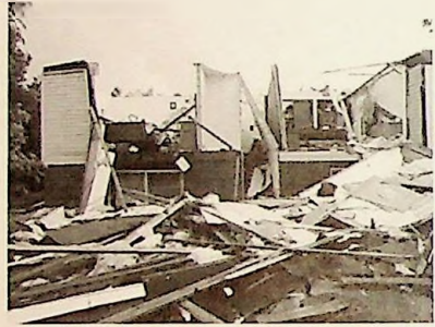
House that was damaged by tornado Photo property of the Kearney Hub, used with permission.
