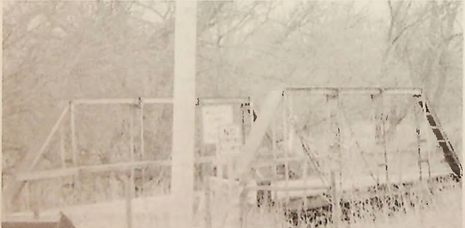
The bridge over Mud Creek on Sweetwater Road, a quarter mile south of Highway 2. The bridge was built around 1909 by the Standard Bridge Company of Omaha.
