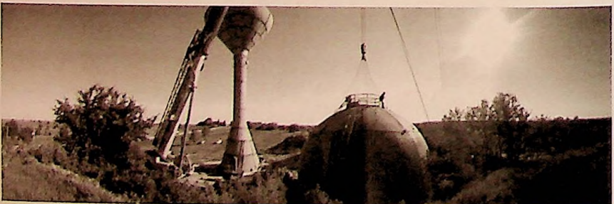
Water Tower Construction— Ravenna, NE (Property of Miller & Associates, used with permission)
